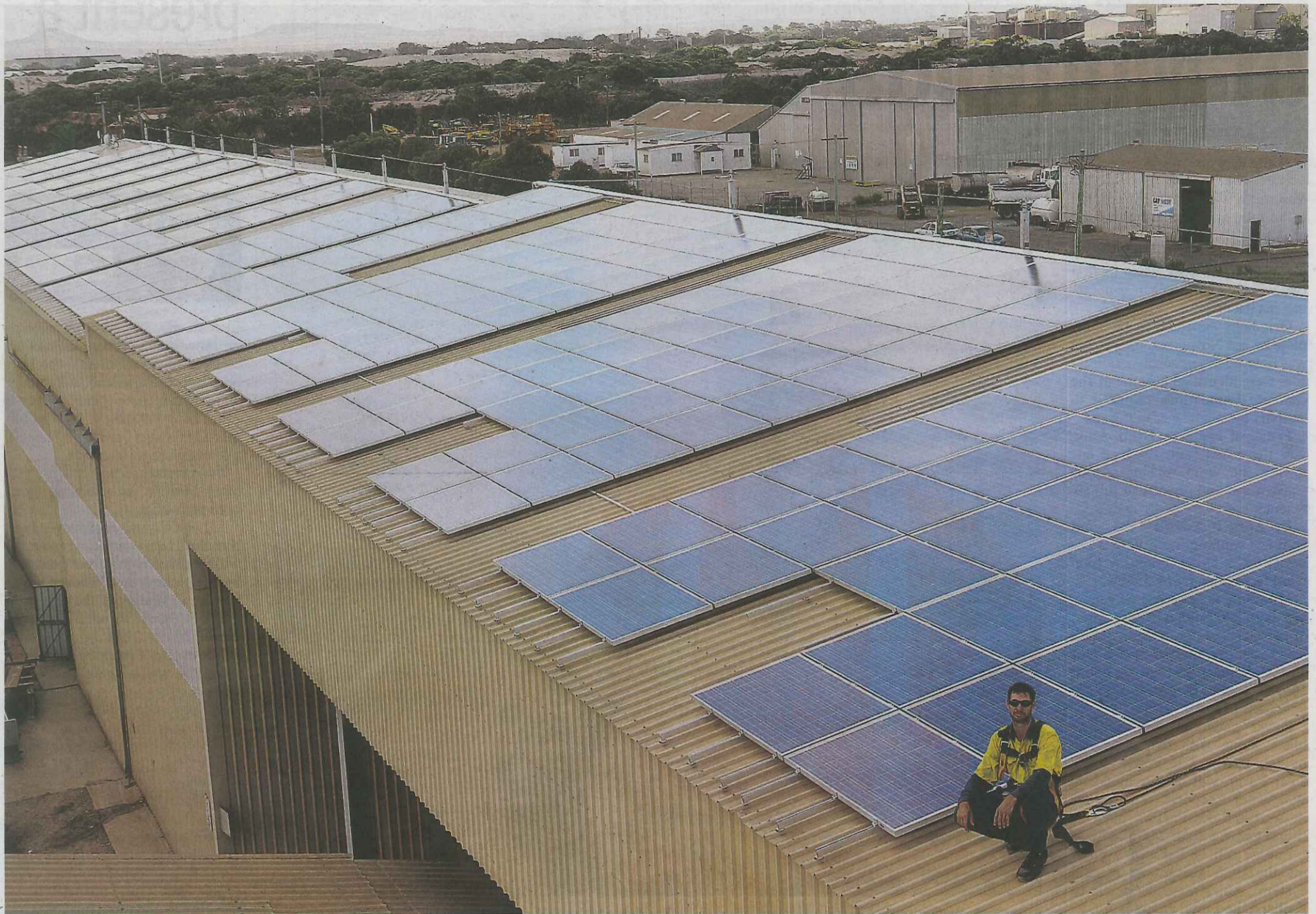
Powering up: Solar panel installer Ryan Daws completes his final check of the big array of solar panels that will drastically reduce DIAB's power bill.
